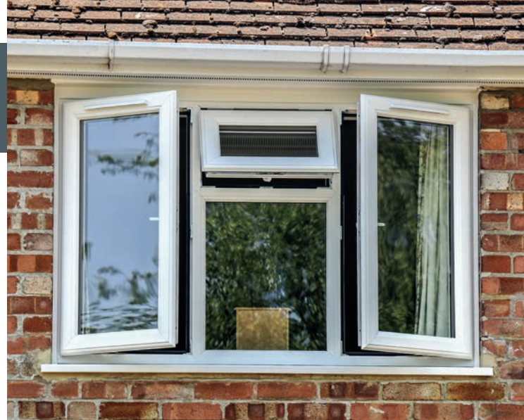
Trickle Vents installed through the window sashes
